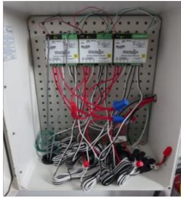
Fig. 2. Installed power meters to measure electricity consumption.
